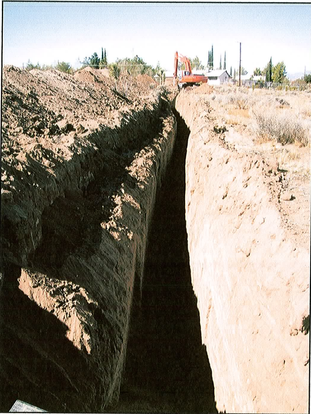
Photo 1: Fault trench No. 2 located across the site traveling in a southwest-northeast direction. A discernable fault trace was located within the trench near the southwest.
